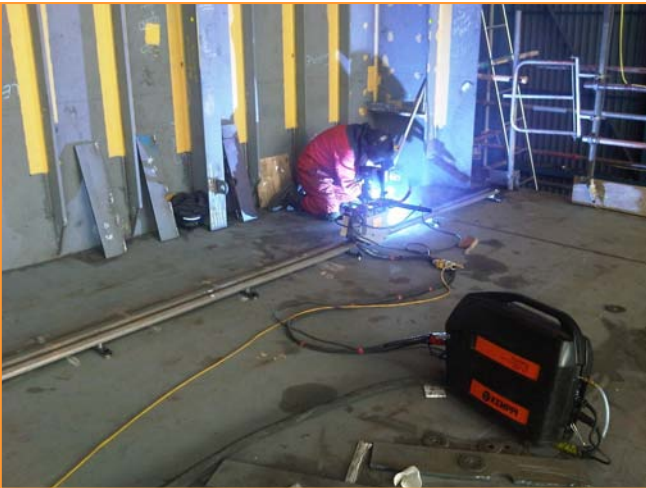
KAT® Welding Carriage System with Oscillator head combination used to complete long continuous weld in the flat position.
