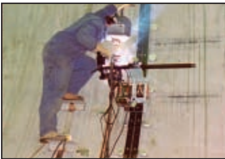
Fig 5. Continuing the weld up the side of the ship in the vertical position using the flexible track.
