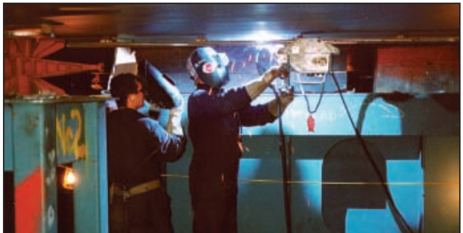
Fig 3. Welding carried out from the outside using a Kat Oscillator and flux cored welding wire in the overhead (PE) position
