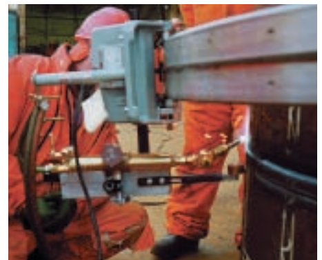
Above: The pipes may also need to be bevelled, as shown, a swivel nozzle makes this easier.
