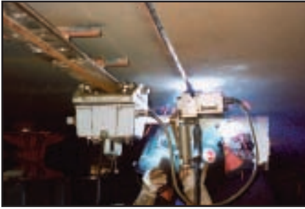
Fig 4. Welding in the overhead position using the Kat Oscillator and flux cored wire
