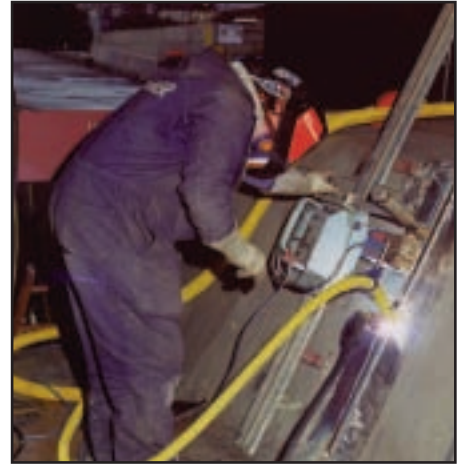
Fig 7. Oscillator welding process in operation joining 316LN stainless steel. This resulted in very high quality welds with minimum surface discontinuities. Furthermore, following the welding operation the Kat Oscillator track could be used for mounting an X-ray head for NDT inspection purposes
