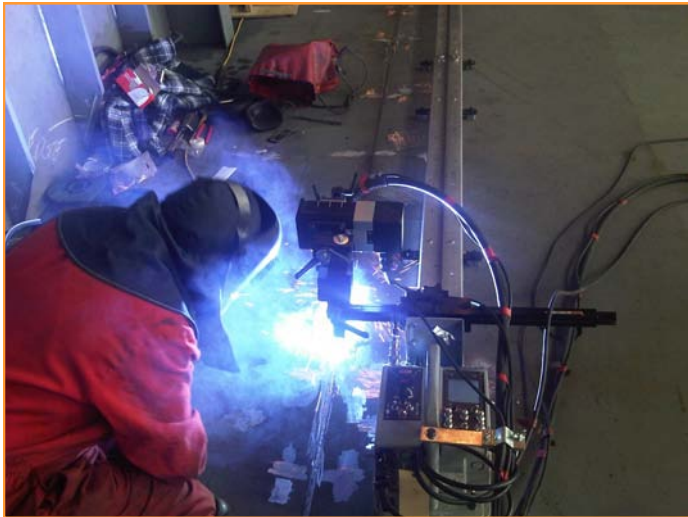
KAT® Welding Carriage System with Oscillator head combination used on multi weld application for UK Aircraft Carriers.
