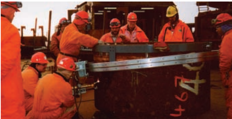
Above: Due to the elliptical path that the Kat takes around the pipe a spring-loaded float is required to maintain the torch height to work. The completed unit is shown here being tested. Note how the track ring is mounted to the steel band.
